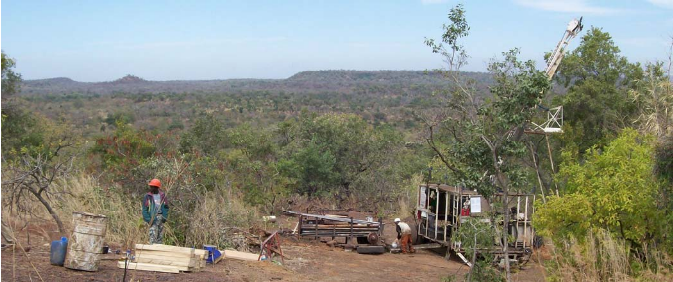
Fig. 2 Diamond Drill Rig at the Diba Target (volcanic plug on horizon above worker with orange hat) Source: Analyst
